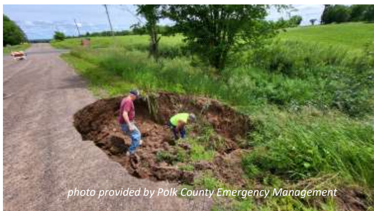
Recent road washout in the Town of Clam Falls following a heavy rain.
